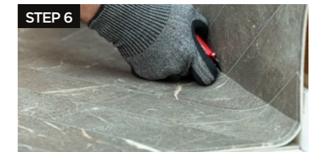
With the material now lying flat around the fittings and corners, the final cutting along the wall lengths can be carried out.
